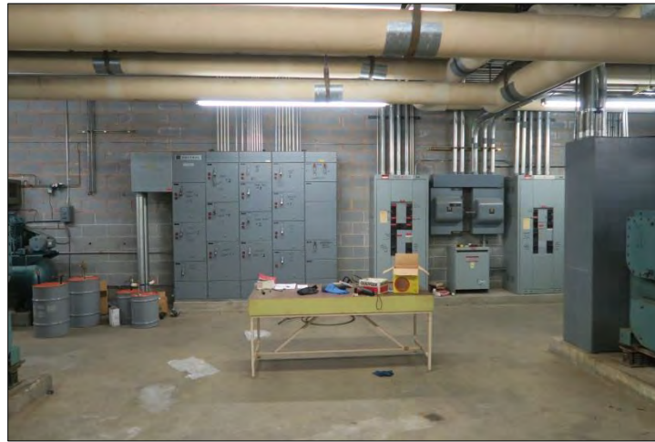
Electrical panels in the penthouse mechanical room
