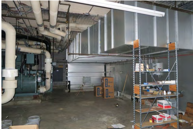
One of three air handlers in the mechanical penthouse
