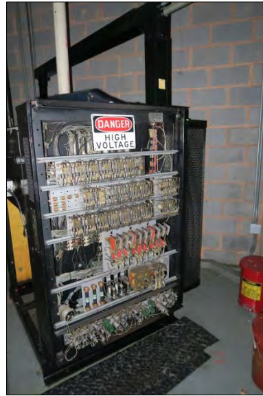
Controls for glass elevator
