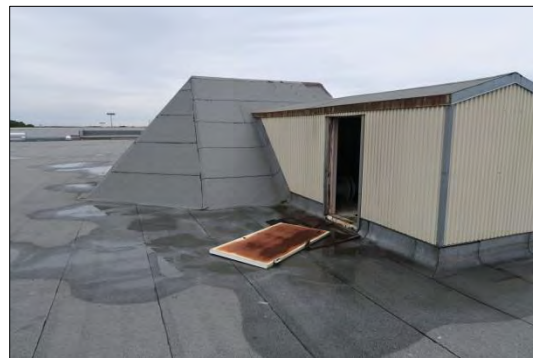
Roof at skylight with some ponding
