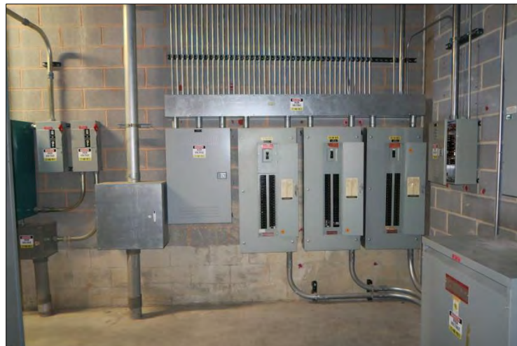
Typical distribution panels & transformers
