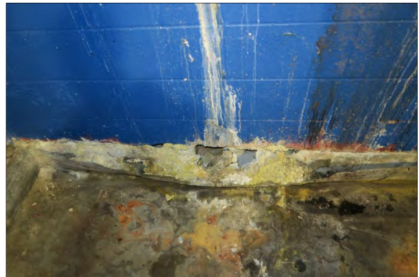
Foundation damage at battery area
