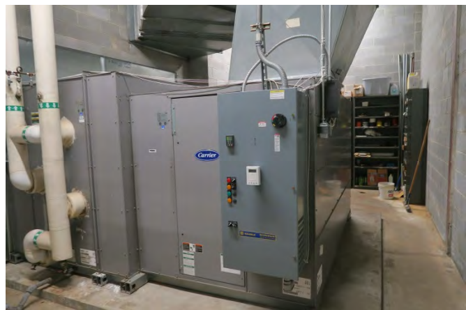
One of three main air handlers
