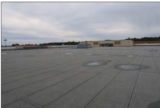
Roof with some ponding
