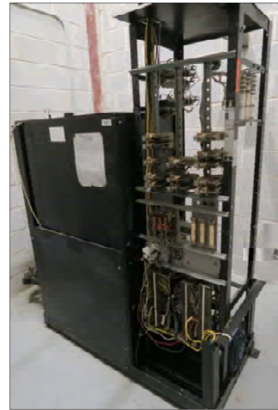
Controls for passenger elevator
