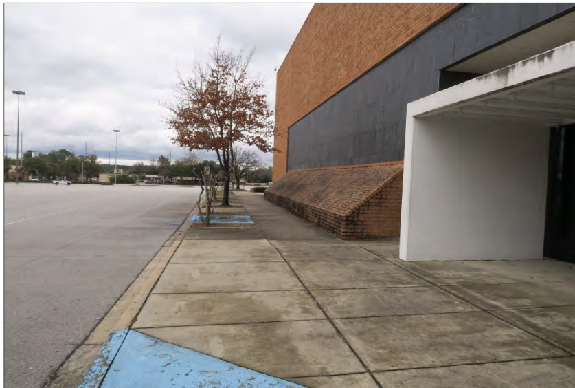
Brick exterior with some evidence of water issues
