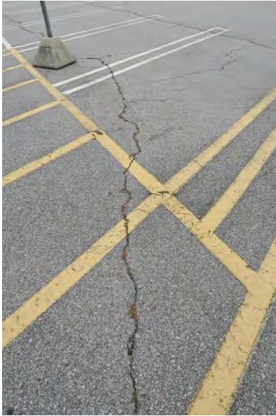
Typical cracking in pavement
