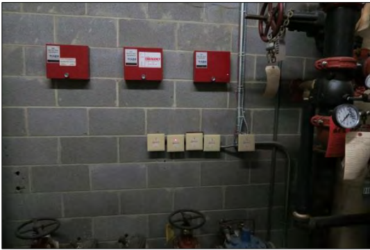
Part of the fire alarm system
