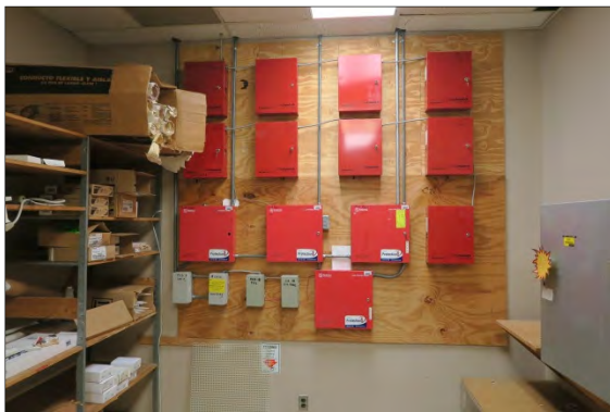
Fire alarm distribution panels
