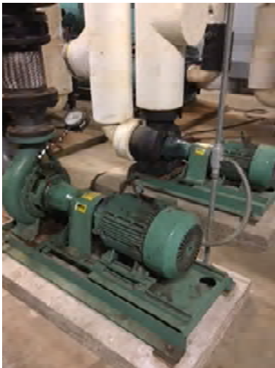
Circulation pumps in the mechanical penthouse
