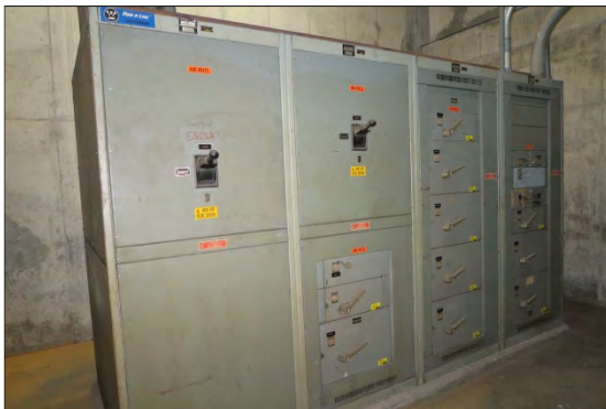
Main switch gear
