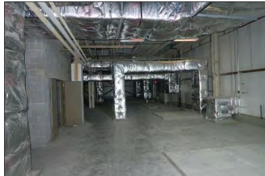
Ductwork from the HVAC Units to the tenant space
