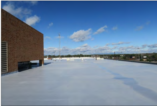
Roof with some ponding
