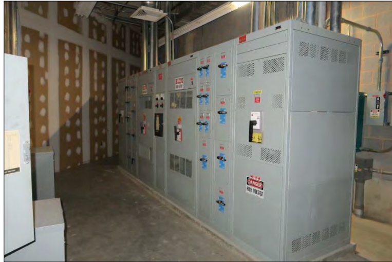
Main switch gear
