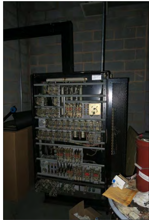
Controls for freight elevator
