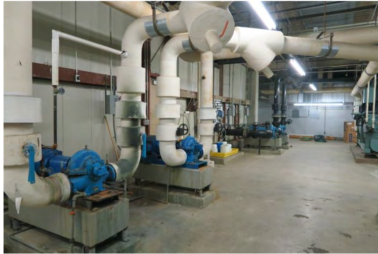
Circulating pumps in the mechanical penthouse
