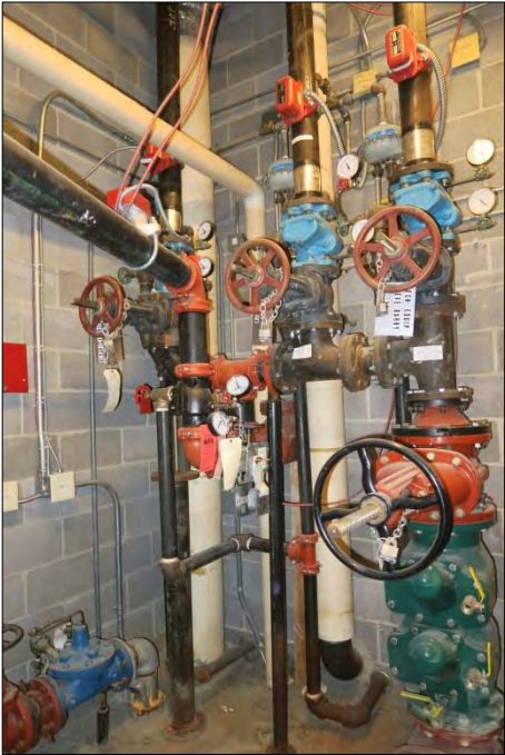
Piping in the fire sprinkler control room
