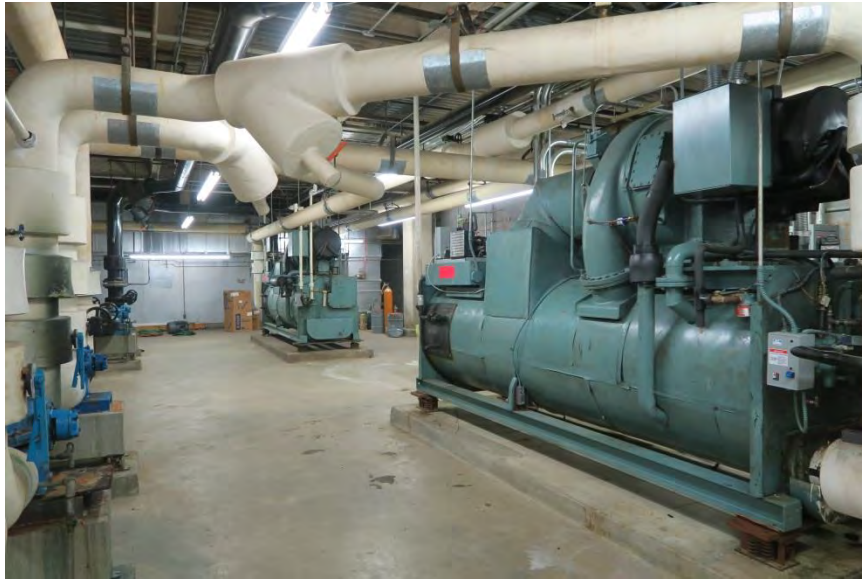
Chillers (1 and 2) in mechanical penthouse
