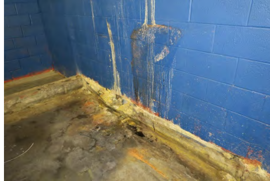
Battery acid damage in auto area
