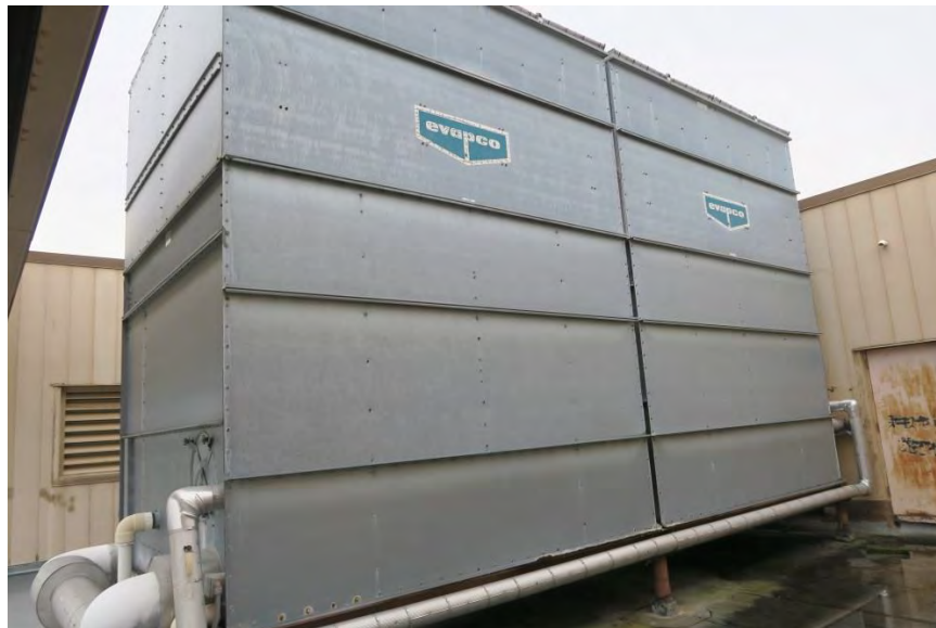
Cooling tower on roof
