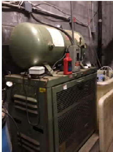
Compressor for pneumatic control system
