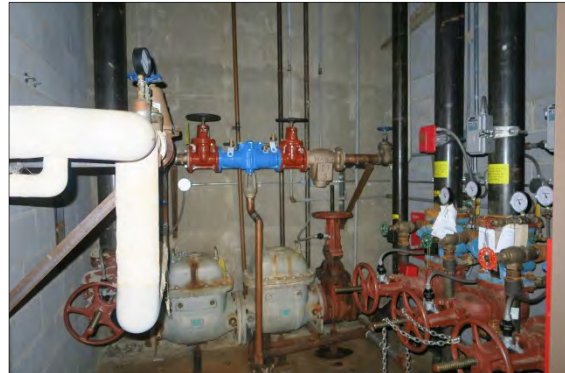
Main domestic water & fire line with back flow preventers
