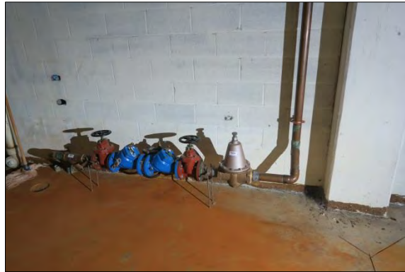
Main domestic water line with back flow preventers
