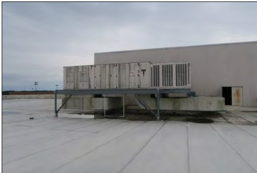
Typical HVAC unit located on the roof
