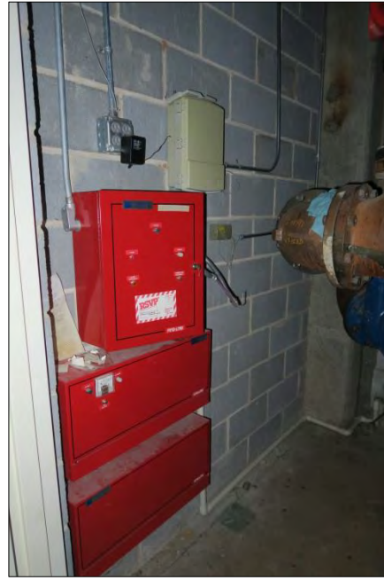
Fire alarm panels in the sprinkler room
