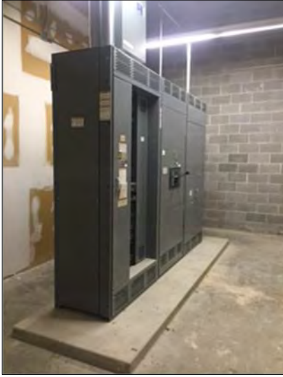
One of the primary switchgear
