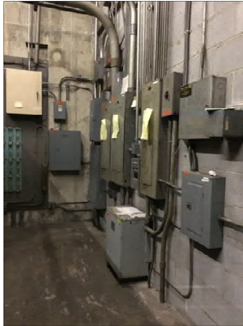
Typical distribution panels & transformers
