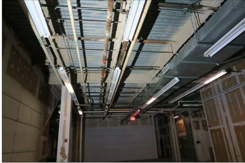
Typical structure (beams and columns with metal deck)- shown in storage area
