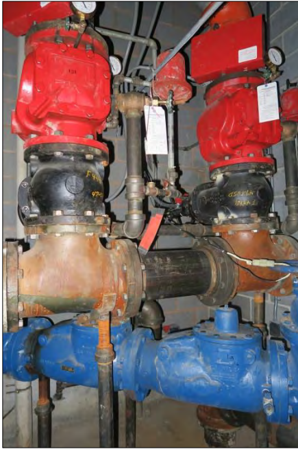
Fire sprinkler room
