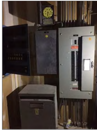
Example of electrical distribution panel
