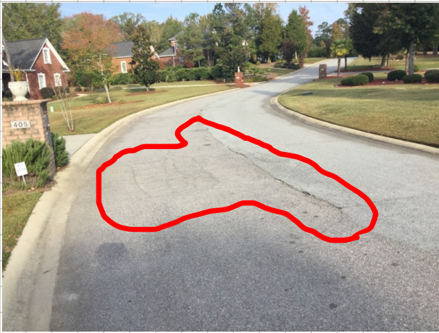
Potholes heavy alligator cracking and dips and ruts have been found on both outbound side and inbound side at the crown of the road proximately 21' x 12'. Location is address 405
