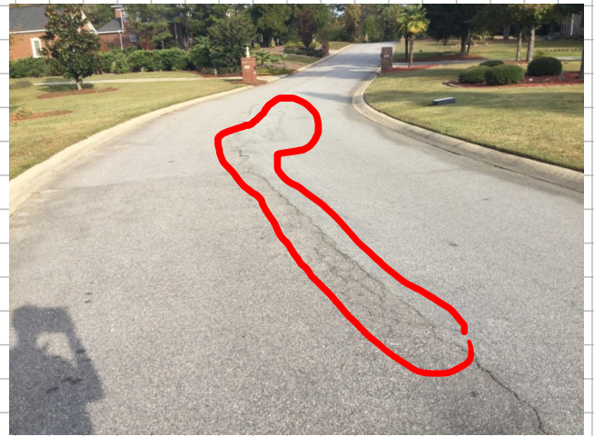
Alligator cracking found at crown of road approximately 45'x2'. Potholes are you there starting to form or have formed within this alligator cracking
