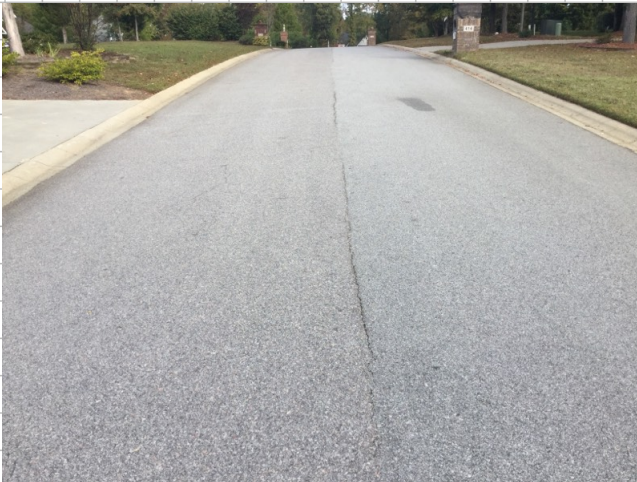
Approximately 142' of cracking down crown of road starting at address for 413 to 419
