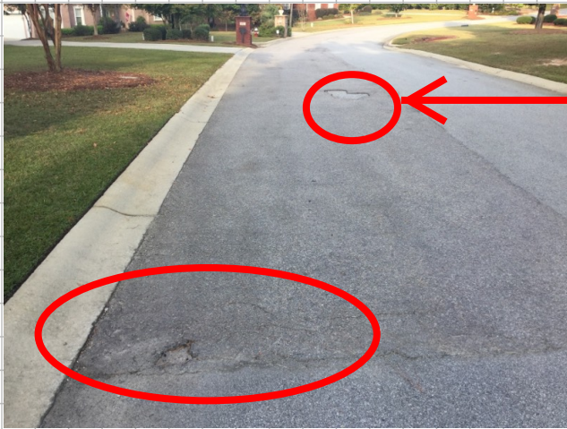
Small pothole right side of outbound lane approximately 8". Alligator cracking around the pot hole area approximately 6' x 1.5'
