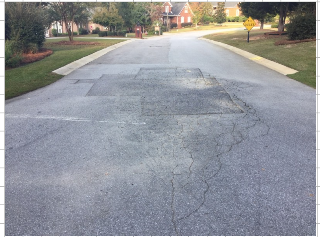
Heavy damage on at start of road alligator cracking, dipping and potholes (36' x15')
