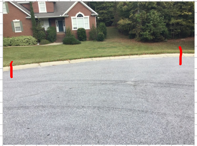
This location of curbing cul-de-sac is approximately 24' in length damage curb also evidence of birdbath in location.
