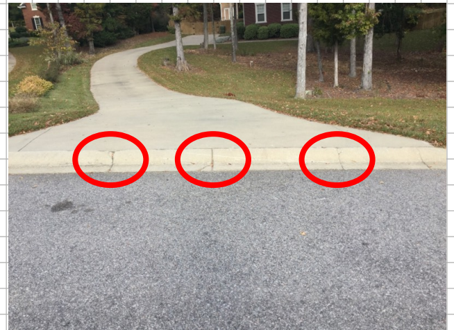
Three locations and curb where pieces are broken have either come out or about to come out
