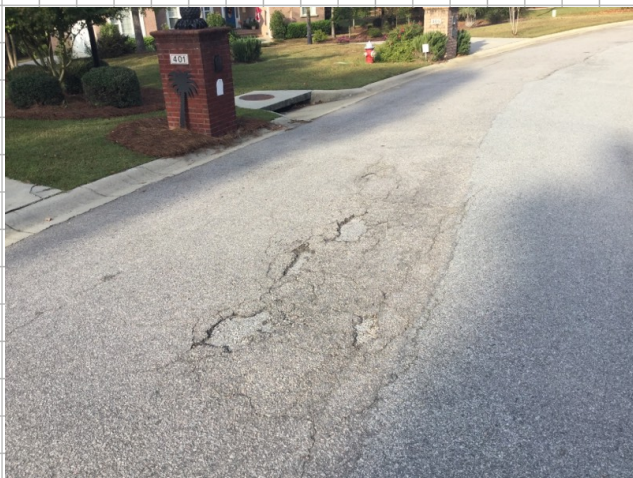
Five potholes starting in alligator cracking approximately 3' x 12'
