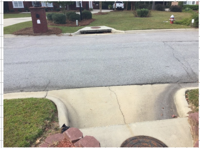
Both storm drain throats on inbound and outbound side of road has cracked throat location is near address 401
