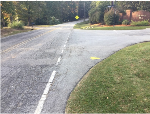
Road damage heavy alligator cracking at intersection with Hiller Road and Ashwood Hill Drive (approx. 78' x 4')
