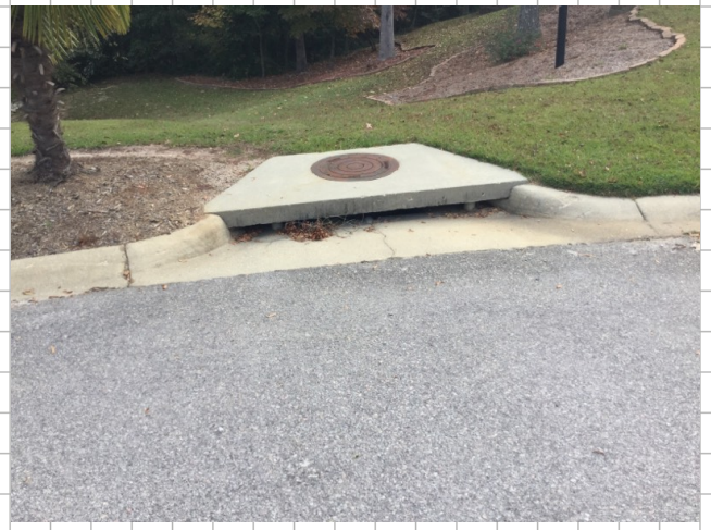
Storm drain in cul-de-sac has cracked throat
