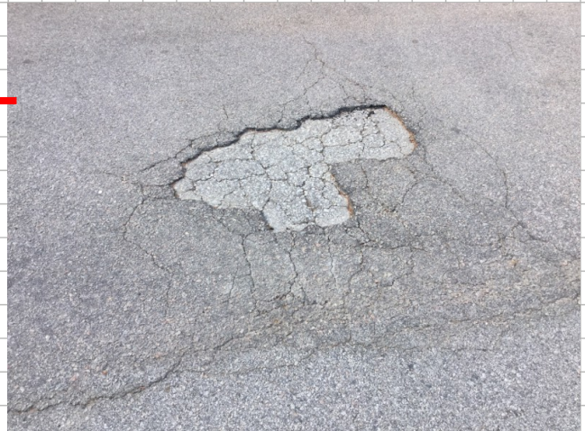
Pothole and outbound lane on left side approximately 2' x 1.5', heavy cracking with in pothole and additional alligator cracking outside a pothole approximately 4' x 5'
