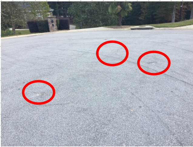
Surface damage found in cul-de-sac. Three locations found that are starting to form potholes (1' diameter)
