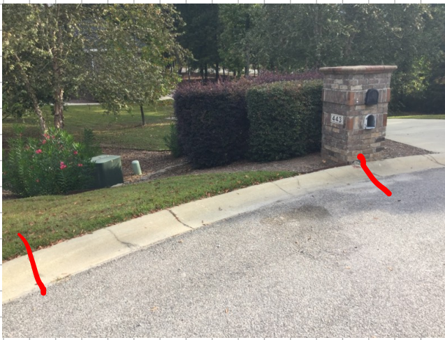
Second location in cul-de-sac with curb damage near address 443, approximately 15', evidence of birdbath also found
