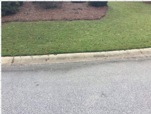
12' section of curb with cracking in large pieces of concrete broken out of curb
