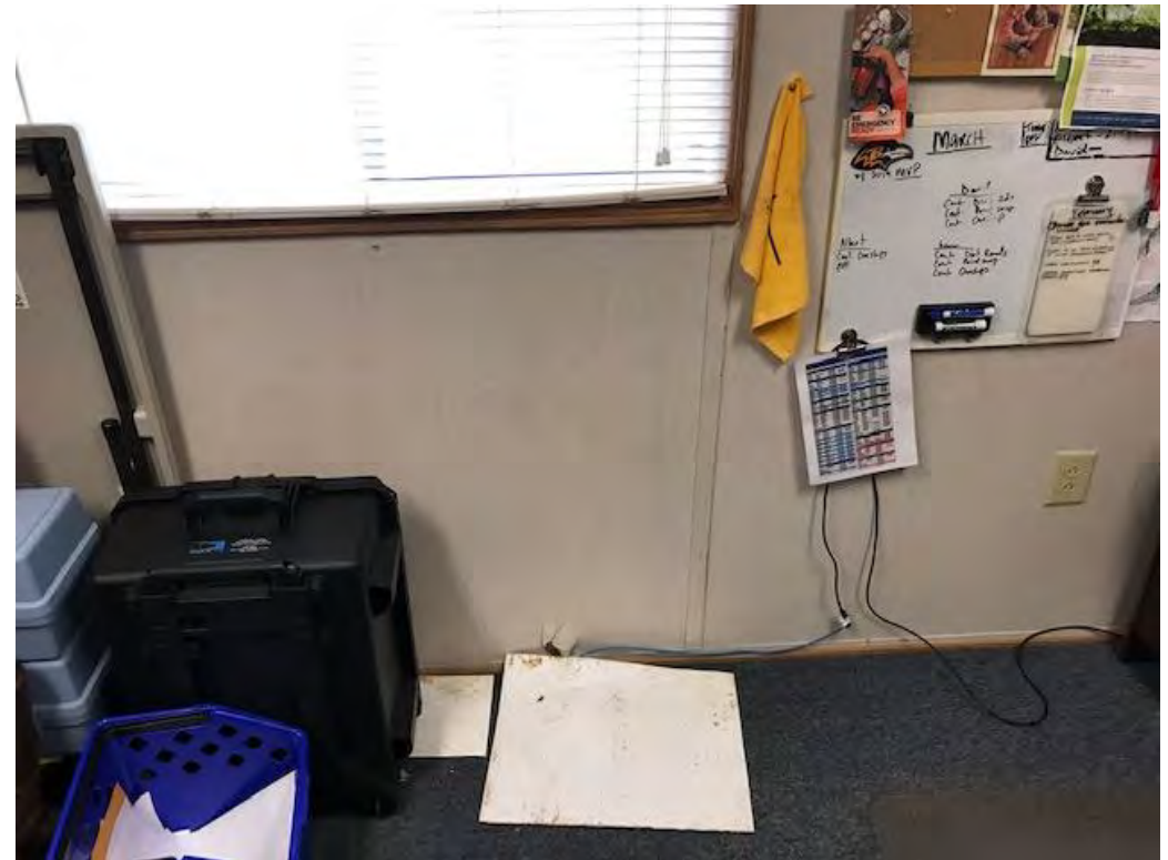
Interior view of absorbent pad next to leaking window.
