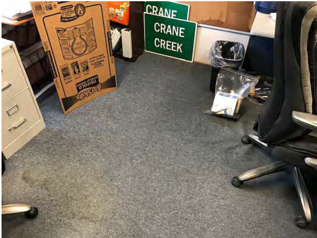
Interior view of carpet discoloration from the leaking roof.
