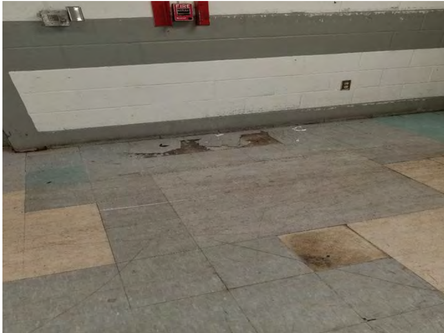
Floor in Need of Replacement
