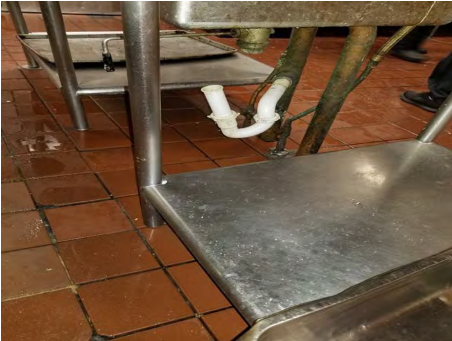
MISSING CONNECTIONS TO SINK
