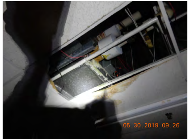
120. Ceiling mount air handler
