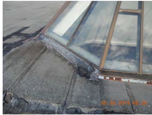
Skylight frame, caulk
