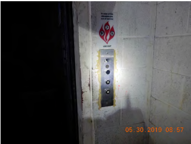
179. Freight elevator controls
