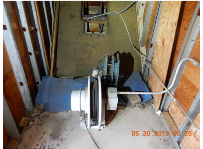
166. Material lift, roof penthouse
