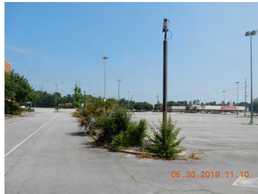
Site lighting, uplight, landscape island
