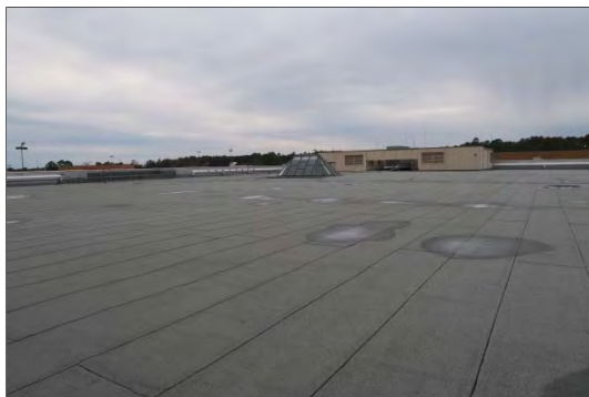
Roof with some ponding
