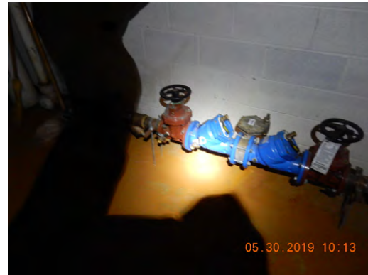
Water service backflow preventer, piping
