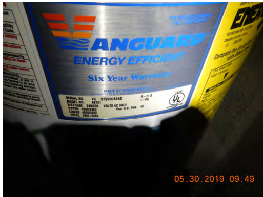
Water heater tag
