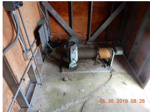
Material lift winch
