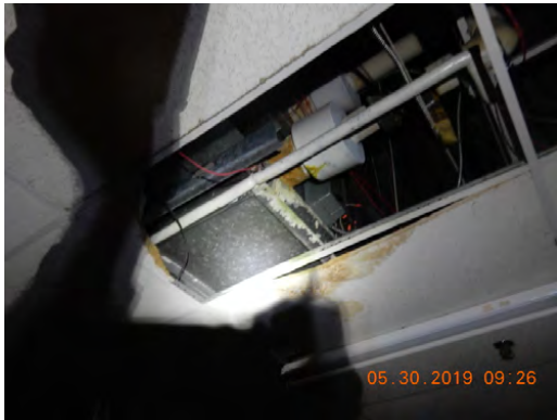
Ceiling mount air handler
