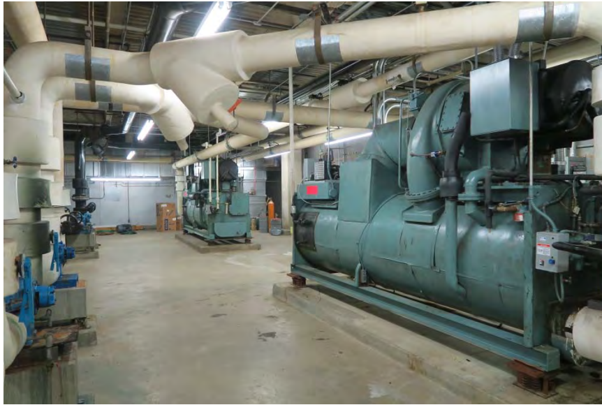
Chillers (1 and 2) in mechanical penthouse
