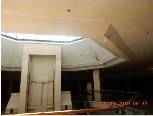
Skylight, water stain
