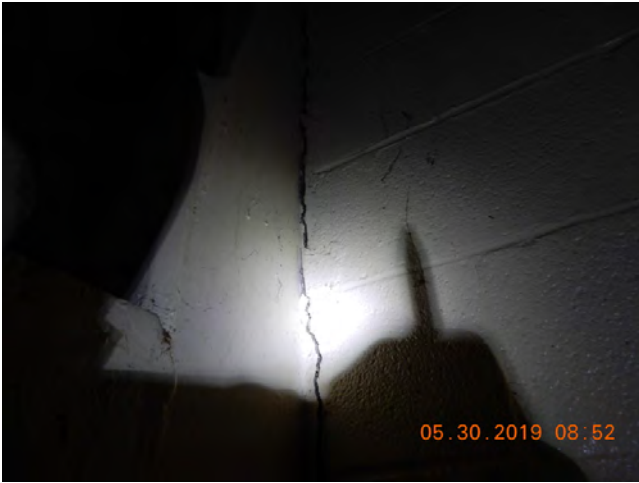
125. Crack at column/corbel, NW stair at roof
