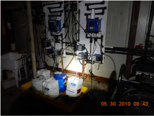
137. Chiller water treatment
