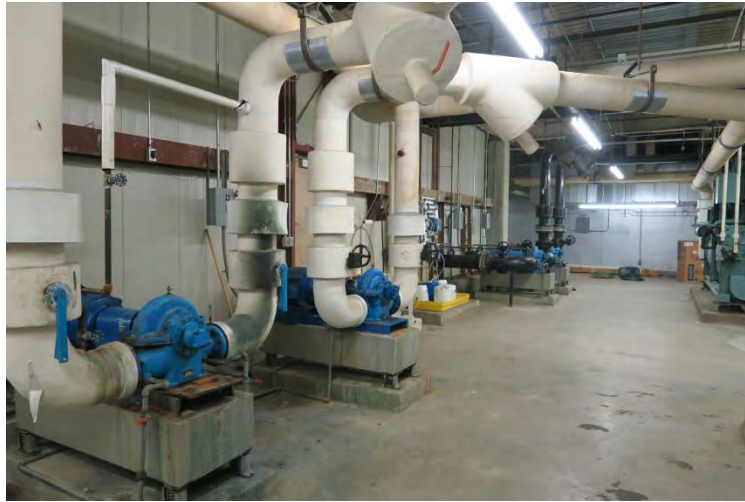
Circulating pumps in the mechanical penthouse
