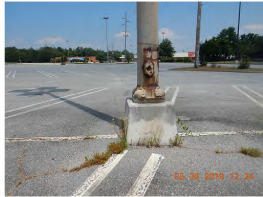
Site lighting pole corrosion
