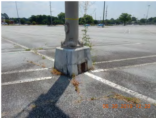
Site lighting pedestal damage
