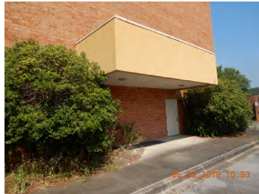
Soffit mounted fixtures
