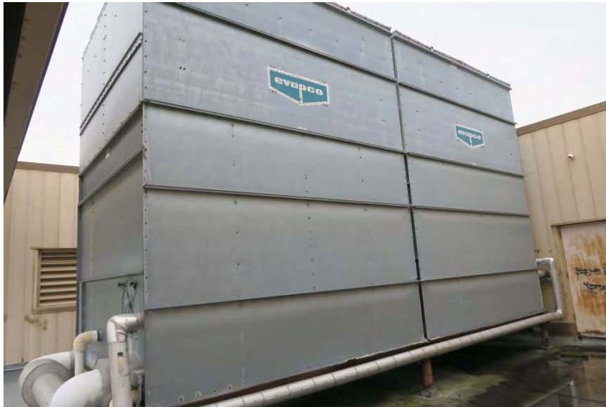
Cooling tower on roof
