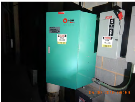
Generator transfer switch
