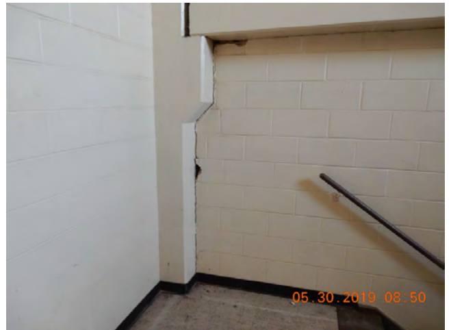
128. Crack, NW stair
