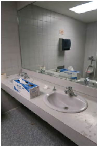
Typical double sinks
