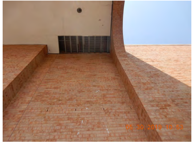
50. Soffit lighting, cladding
