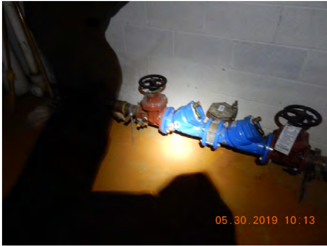
73. Water service backflow preventer, piping
