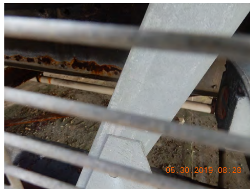
Cooling tower corrosion
