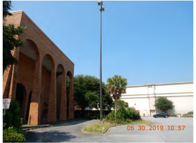
38. Site lighting, landscape island
