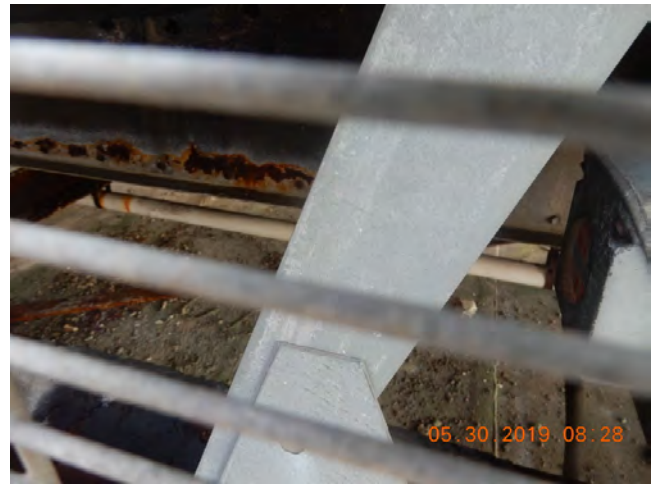
162. Cooling tower corrosion
