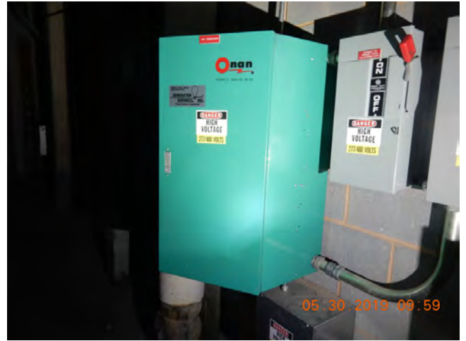
82. Generator transfer switch
