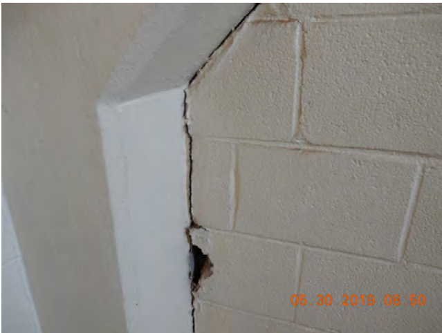
127. Crack, NW stair
