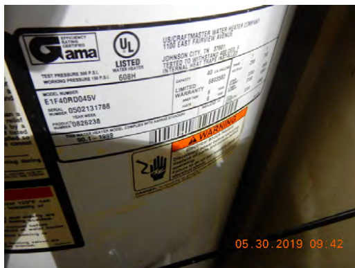
Water heater tag
