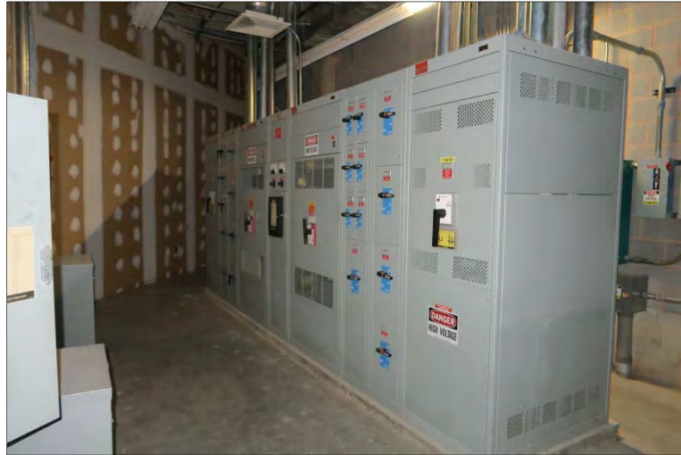
Main switch gear
