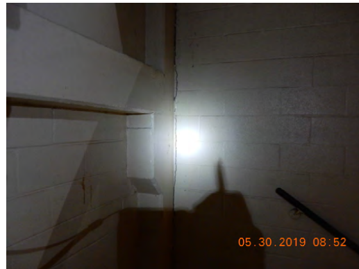
Crack at column, NE stair
