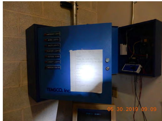
Lighting control panel
