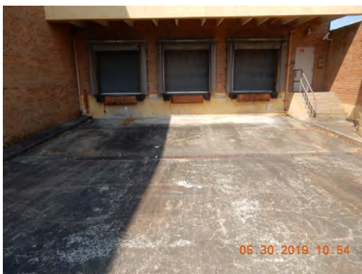
Dock, trench drain
