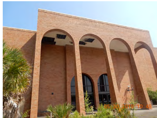
South elevation, soffit damage
