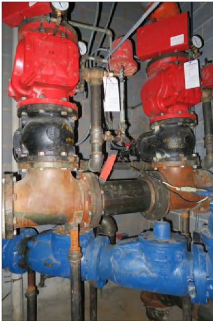
Fire sprinkler room
