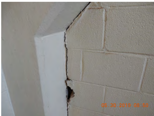
Crack, NE stair
