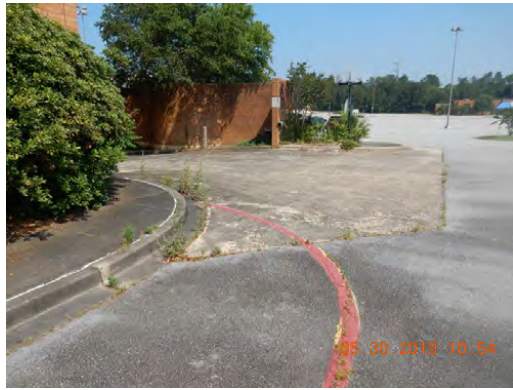
Dock apron damage
