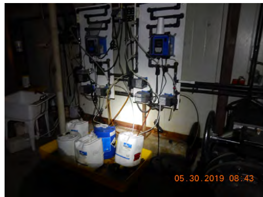
Chiller water treatment
