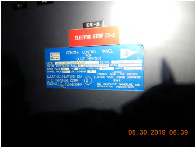
145. Duct heater control
