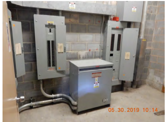
72. Panels, transformer, bearing wall structure
