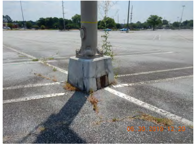
6. Site lighting pedestal damage
