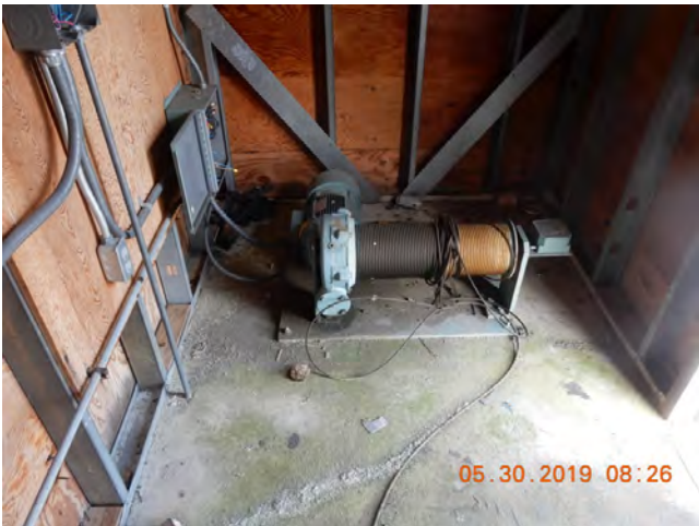
167. Material lift winch
