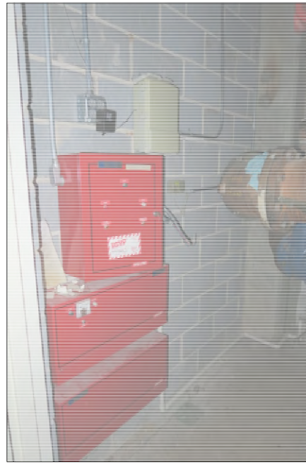
Fire alarm panels in the sprinkler room
