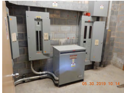
Panels, transformer, bearing wall structure
