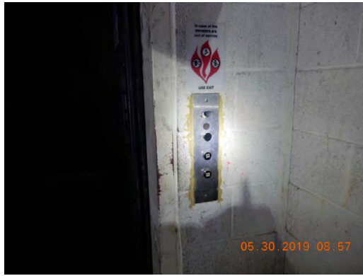
Freight elevator controls
