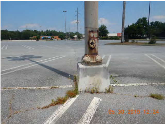
3. Site lighting pole corrosion
