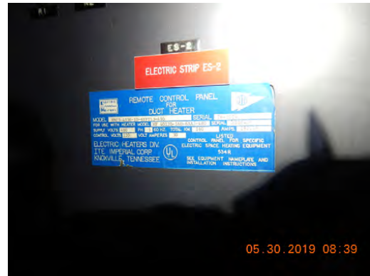
Duct heater control
