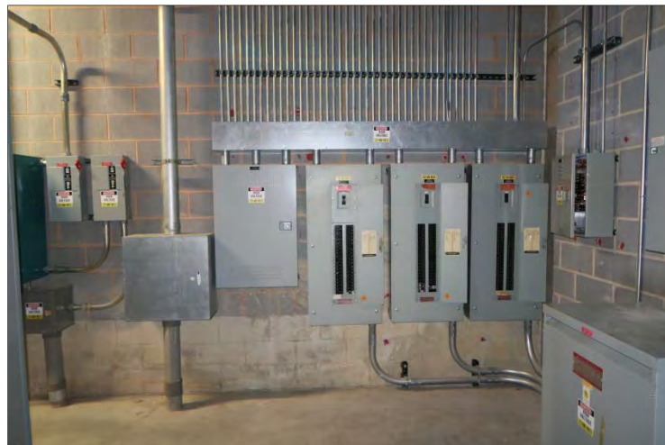
Typical distribution panels & transformers
