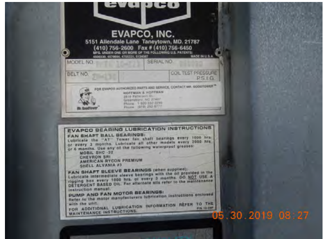
164. Cooling tower tag
