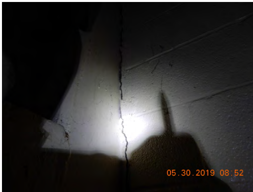
Crack at column/corbel, NE stair at roof
