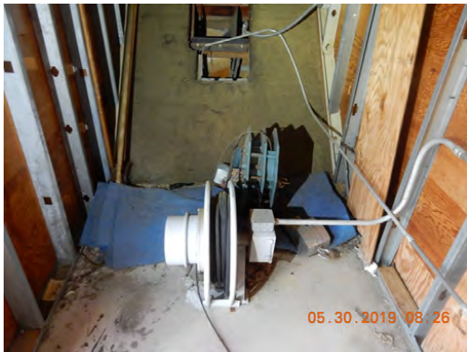
Material lift, roof penthouse
