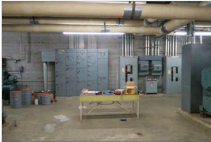
Electrical panels in the penthouse mechanical room
