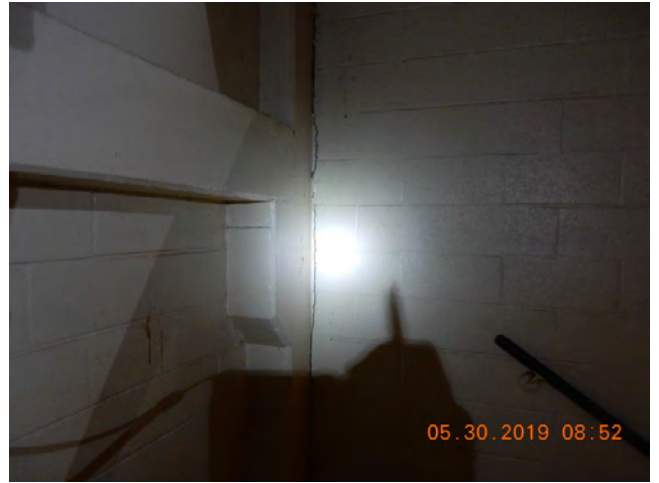
126. Crack at column, NW stair
