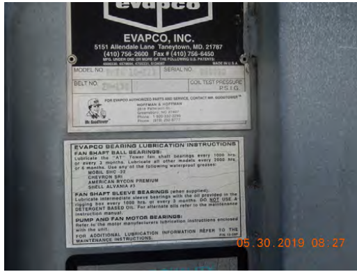
Cooling tower tag
