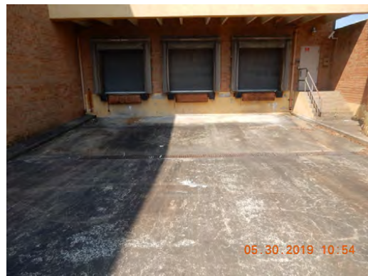
Dock, exterior steps; concrete damage at north dock door
