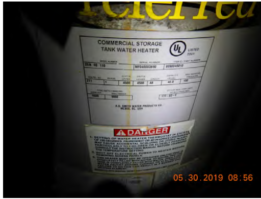
Water heater tag
