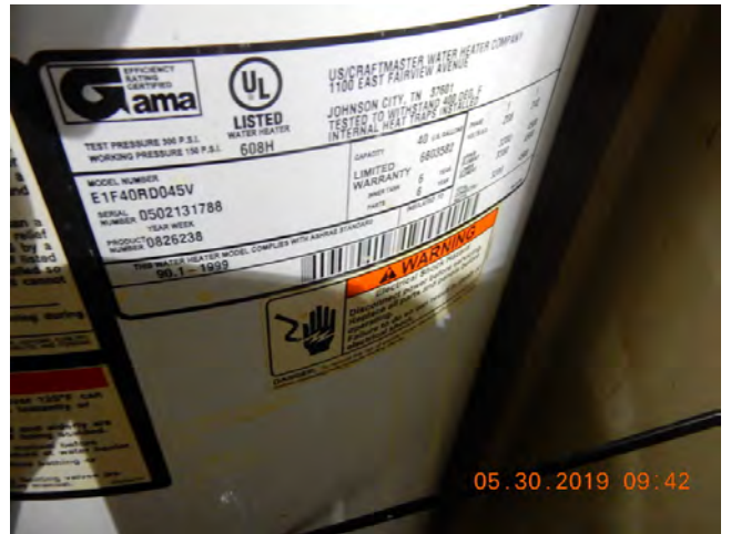
104. Water heater tag
