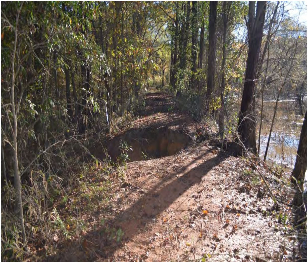
Figure 1: Poorly Maintained Dam with Extensive Tree Growth
