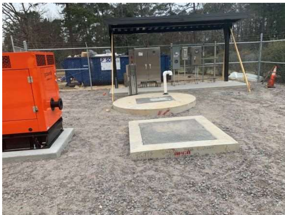
Photo 4: Trotter pump station
