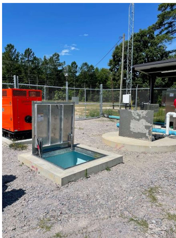
Photo 4: Trotter pump station
