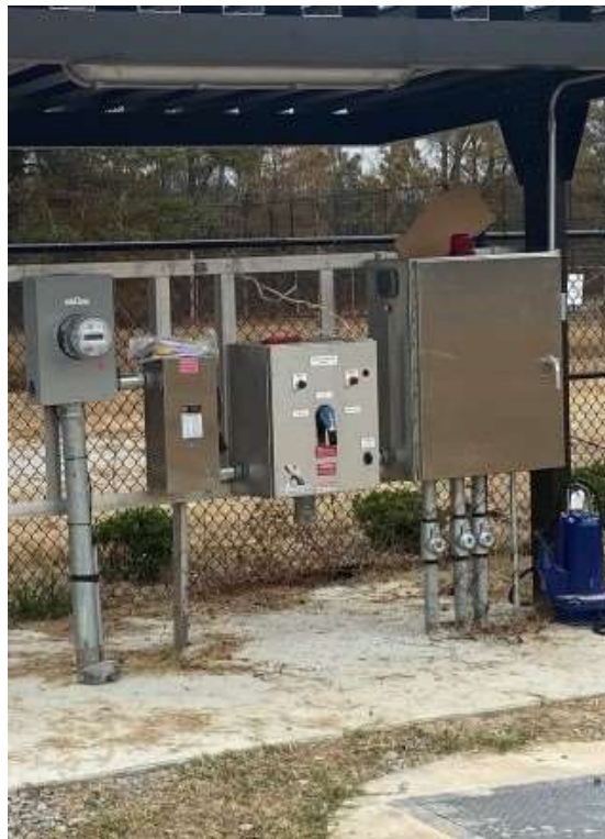
Photo 3: Hopkins Middle Control Panel
